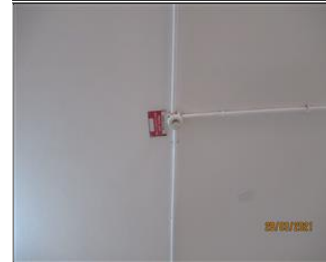
Photo of fire safety equipment Smoke detector.JPG
