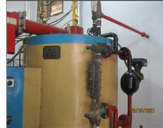
External photo(s) of the production unit(s) Boiler.JPG
