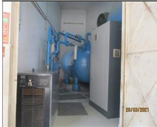
External photo(s) of the production unit(s) Compressor room.JPG
