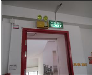
Photo of the inside of the main production hall Exit sign illuminated and emergency exit signage.JPG
