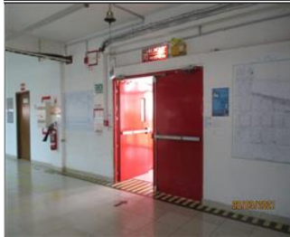
Photo of fire safety equipment Fire Resistance Emergency Exit Door.JPG
