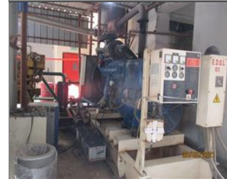
External photo(s) of the production unit(s) Generator.JPG
