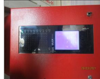
Photo of fire safety equipment Fire control panel.JPG
