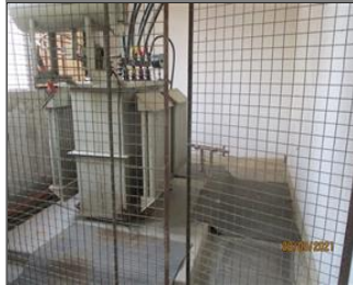
External photo(s) of the production unit(s) Electrical sub-station.JPG
