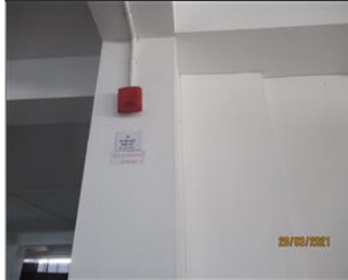
Photo of fire safety equipment Fire alarm bell.JPG
