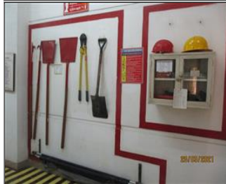
Photo of fire safety equipment Other firefighting equipments.JPG
