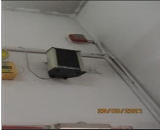
Photo of the inside of the main production hall PA system.JPG
