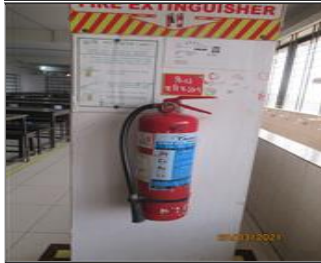
Photo of fire safety equipment Fire extinguisher.JPG
